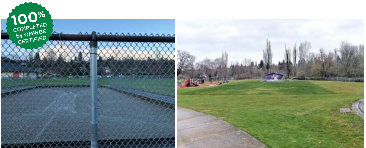
Figure 3: Before and after: the removal of Portland Avenue wading pool was completed in 2022 by Woodland Industries, SBE, as general contractor. Utilization for this project was 100%.
