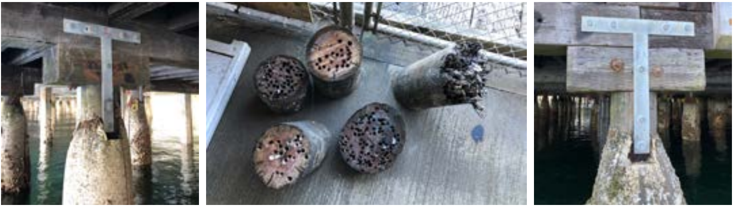
Figure 5: Major renovations to the pier at Point Defiance Marina were completed by American Construction working with Associated Underwater Services, DBE/WBE. MWBE utilization was 10% on this specialized work.
